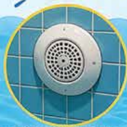
SUCTION OUTLETS Found on the walls of the pool or spa.
